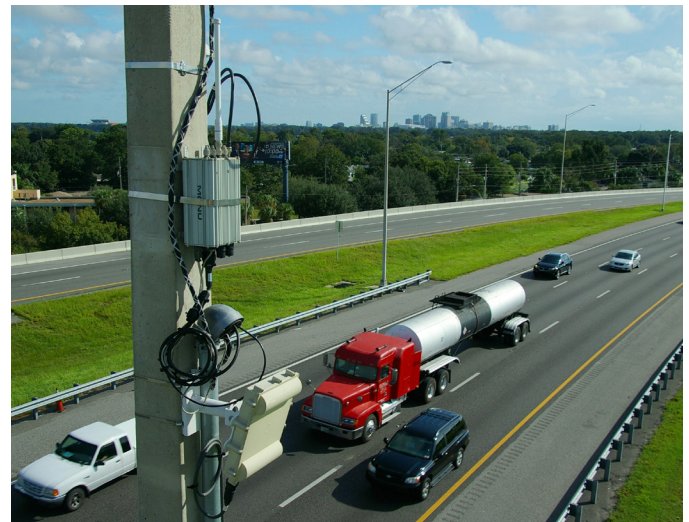
4. Close-up of Roadside Equipment
