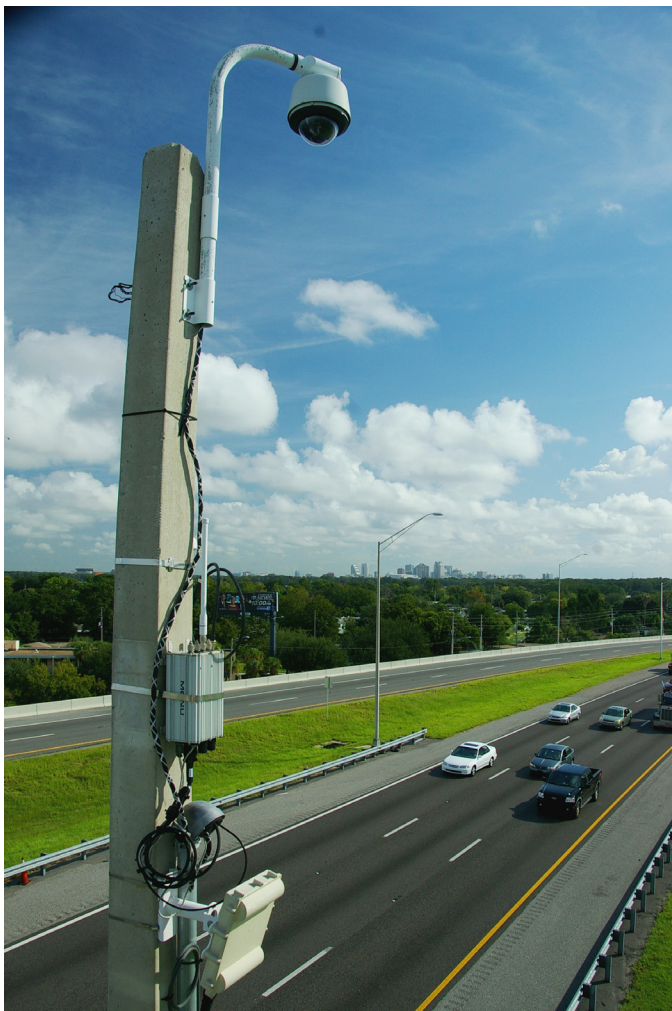
2. Intelligent Transportation System at Work: CCTV Camera, Roadside Equipment and Roadside Sensor
